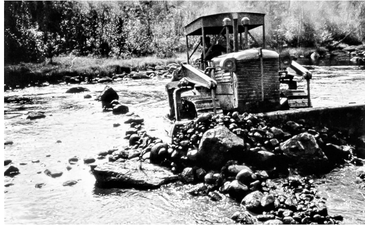
Clearing stones and boulders from a river with the help of a bulldozer to allow easier floating of timber.
